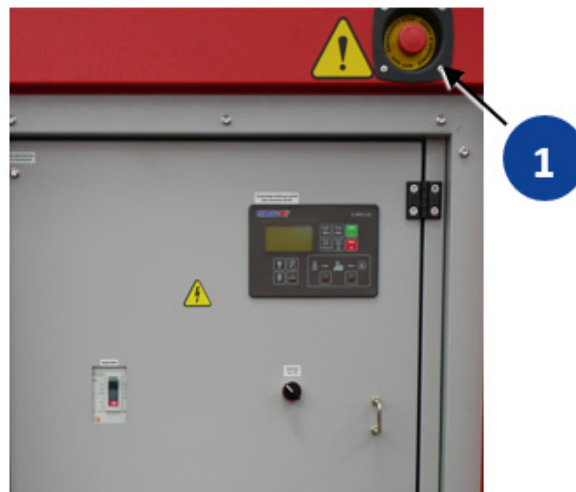
Fig. 7-8 EMERGENCY-STOP smash button
